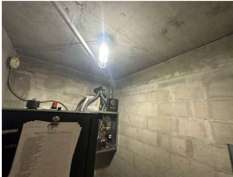
Figure 14: Elevator Mechanical Room, Level 1
